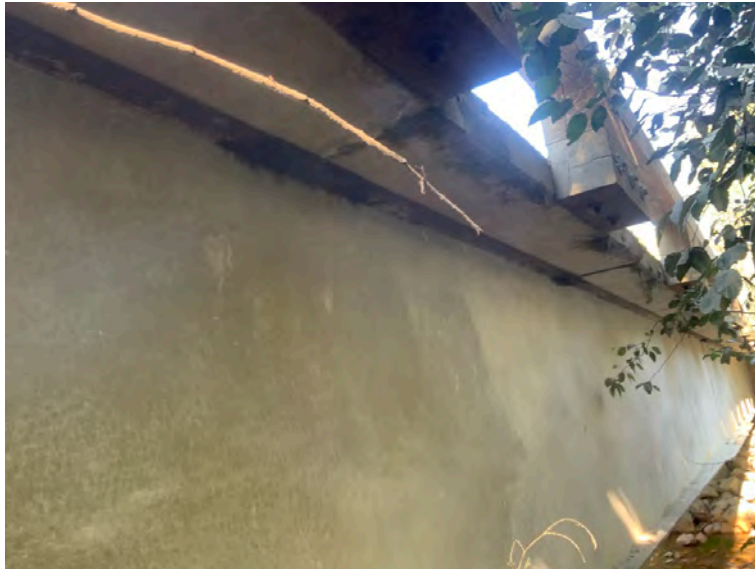
Superstructure, corrosion under deck joints
