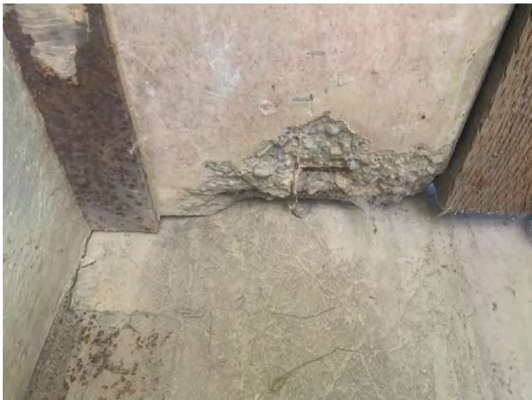
First panel, left bank underside. Rebar showing
